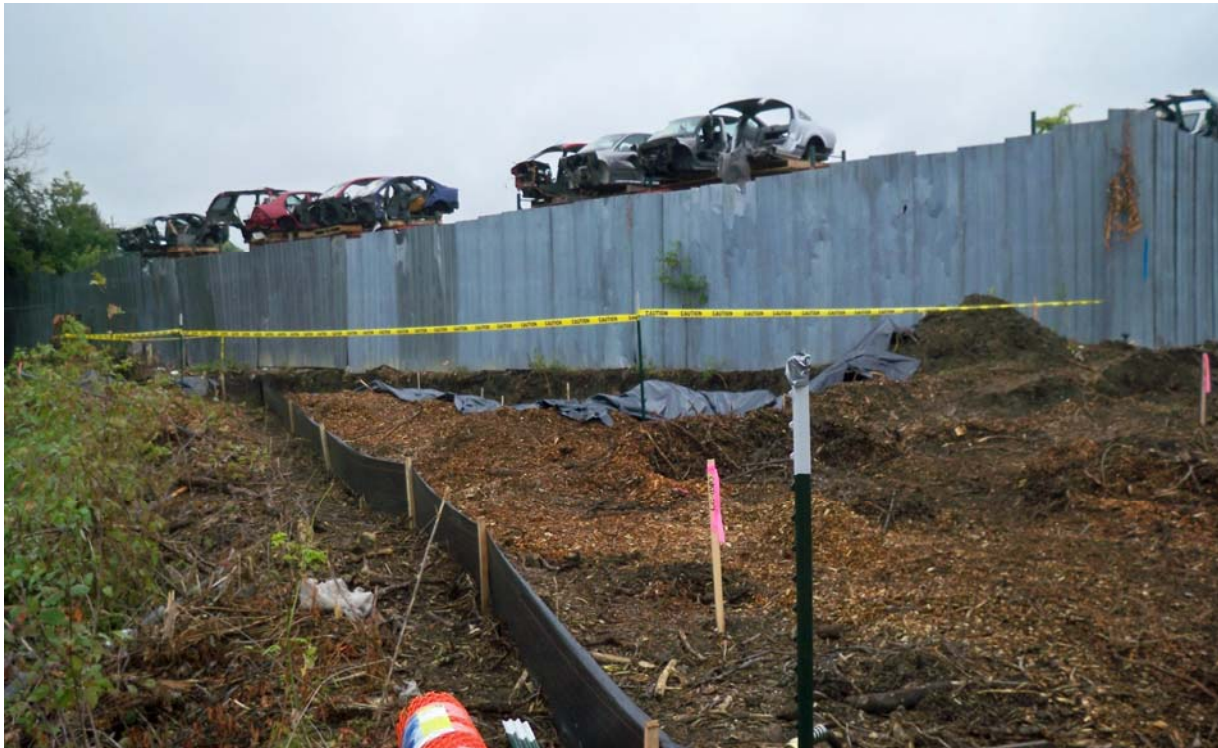
Photo #12: Installed silt fence and caution tape for access control within excavation footprint
