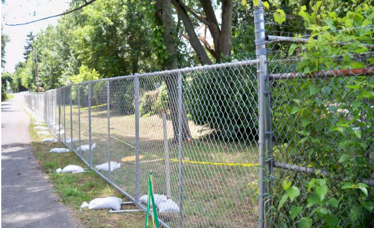
Photo #7: Perimeter fence for access control
