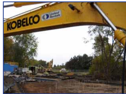
A view of remediation work underway looking toward the south of Haley's Ditch from the north end of the site.
