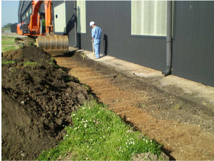
Photo # 1: Facing south the photo depicts excavation activities continuing from the northern section to the southern section.
