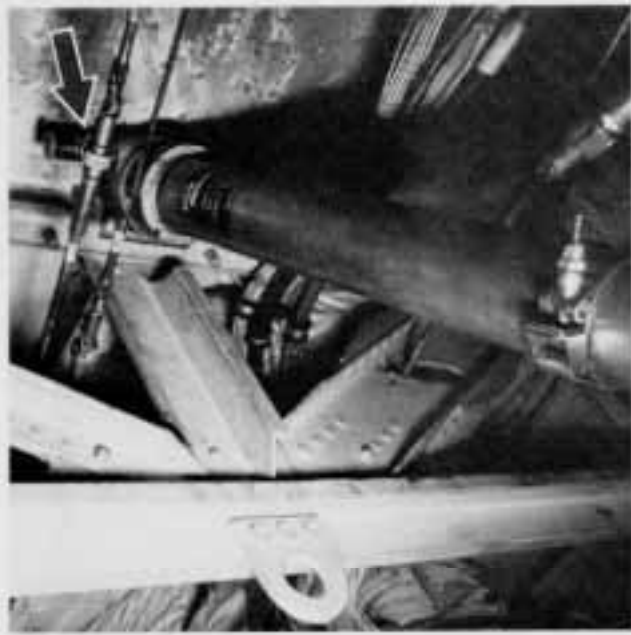
Aft cargo door actuator. Note the protruding bleed valve.
