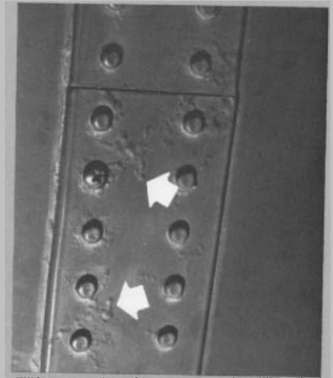
Filiform corrosion often appears as threadlike raised areas under organic coatings.
