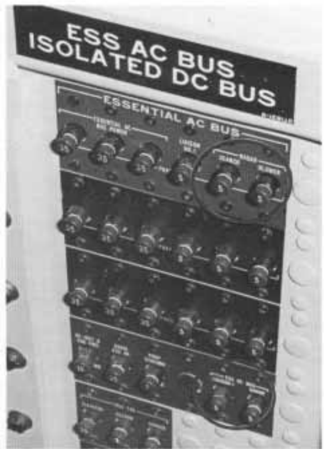
Circuit breakers for the APQ-122 radar.
