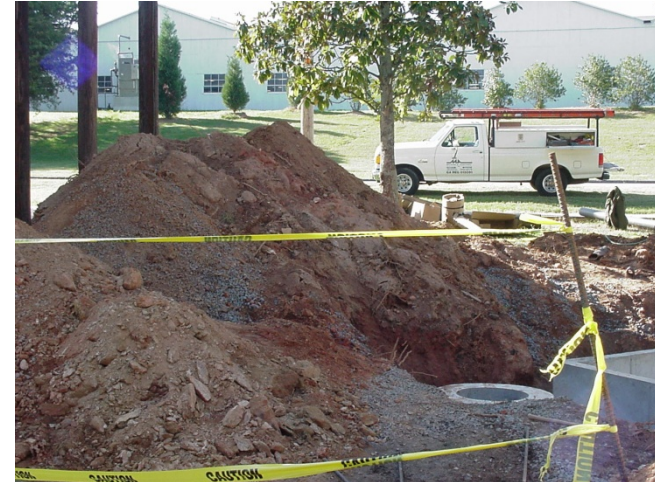
Soil < 2 ft. from excavation
