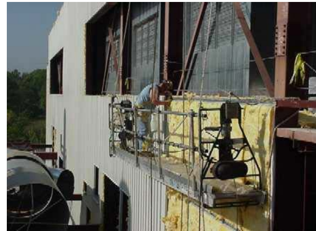
No Fall Protection Equipment
