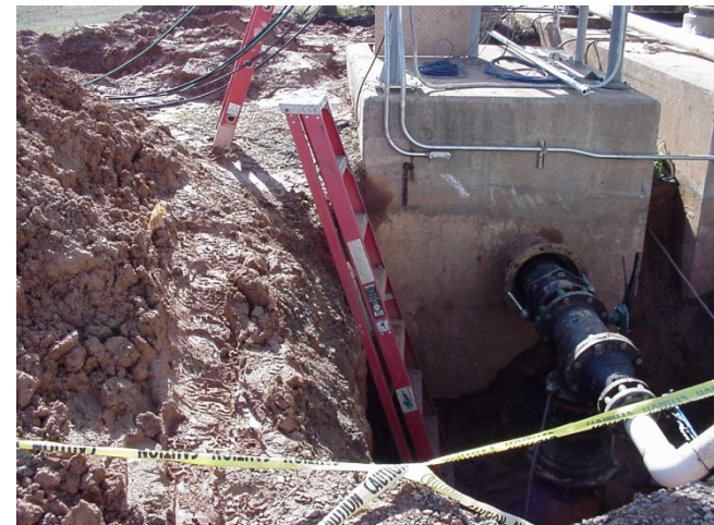
Not properly sloped, benched, etc.
