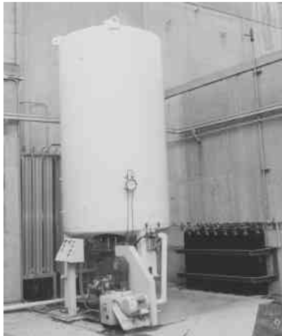
Figure 6-10 High Pressure Nitrogen Gas Facility
