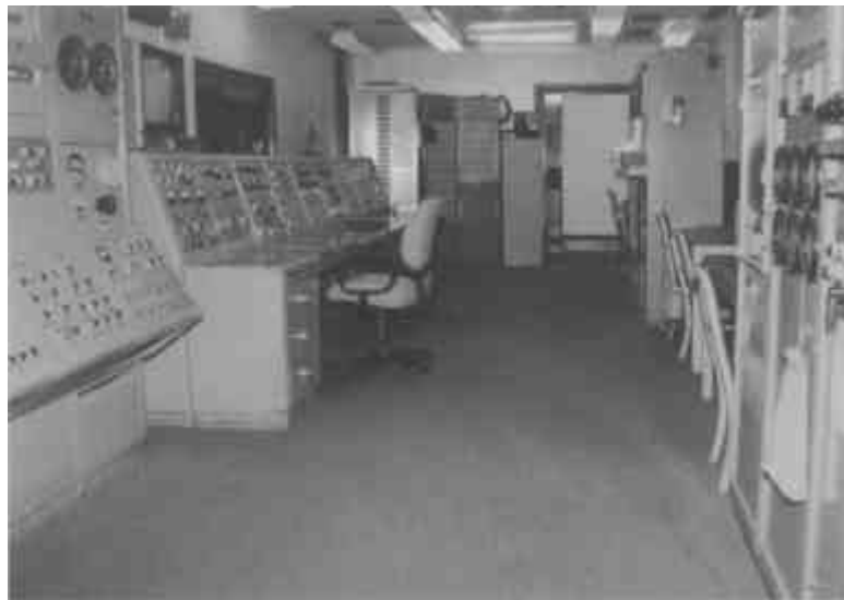
Figure 2-5 Control Room and Data Signal Conditioning and Acquisition System
