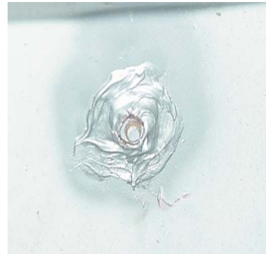
Putty Inside Door / Unusual
