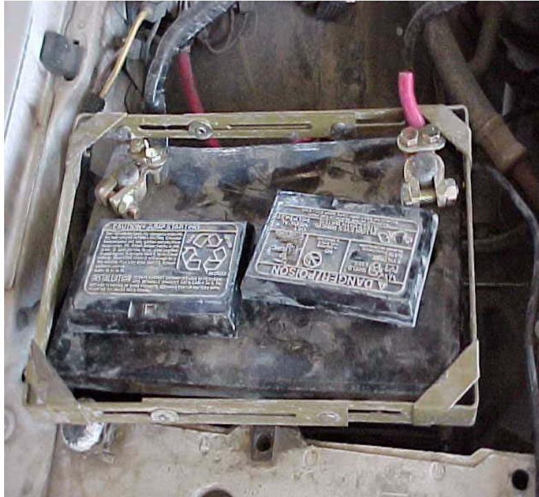
Top Cover Loose / Not Wired
